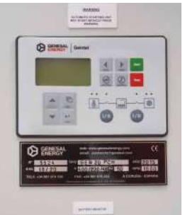
Panel de control
